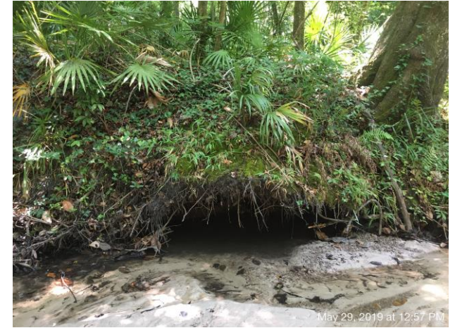
Bank erosion due to excavation on Hogtown Creek
